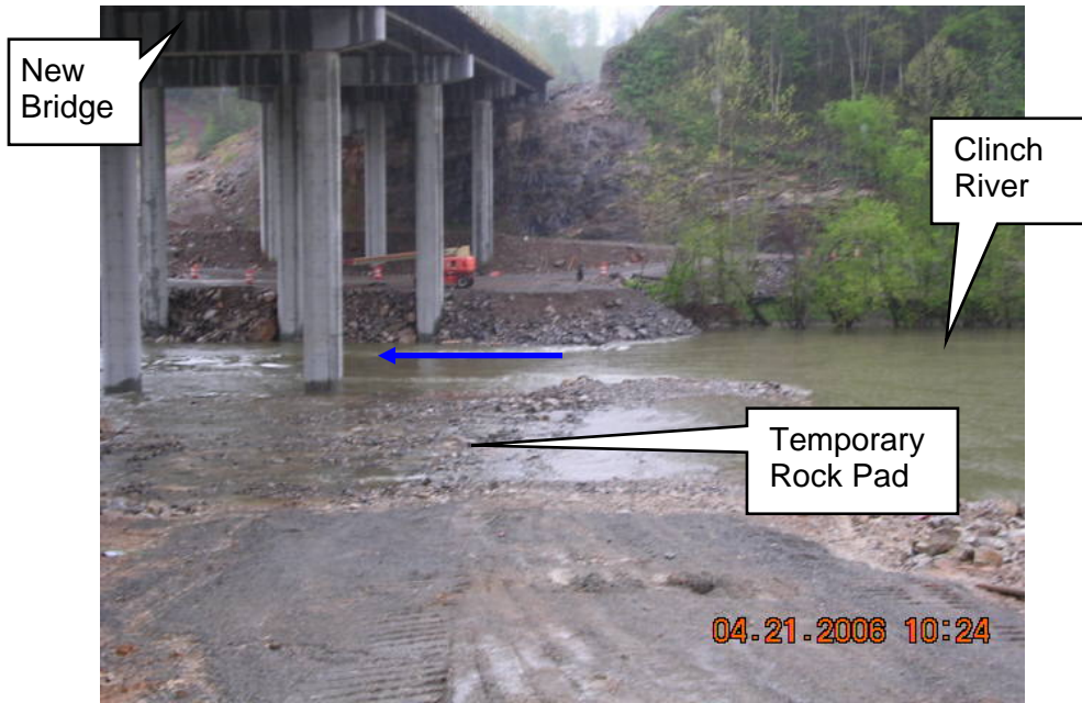
Photo 1. Temporary rock pad for bridge construction at Sta. 3+540 (both sides of centerline). View from south bank of the Clinch River looking northwest.
