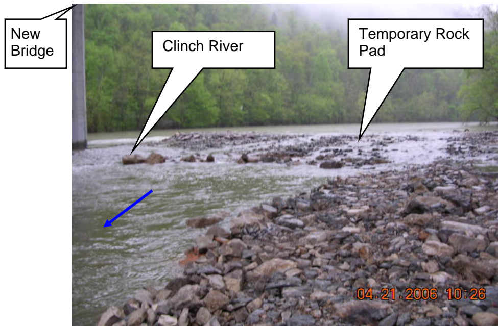
Photo 4. Temporary rock pad for bridge construction at Sta. 3+540 (both sides of centerline). View from south bank of the Clinch River looking northeast.
