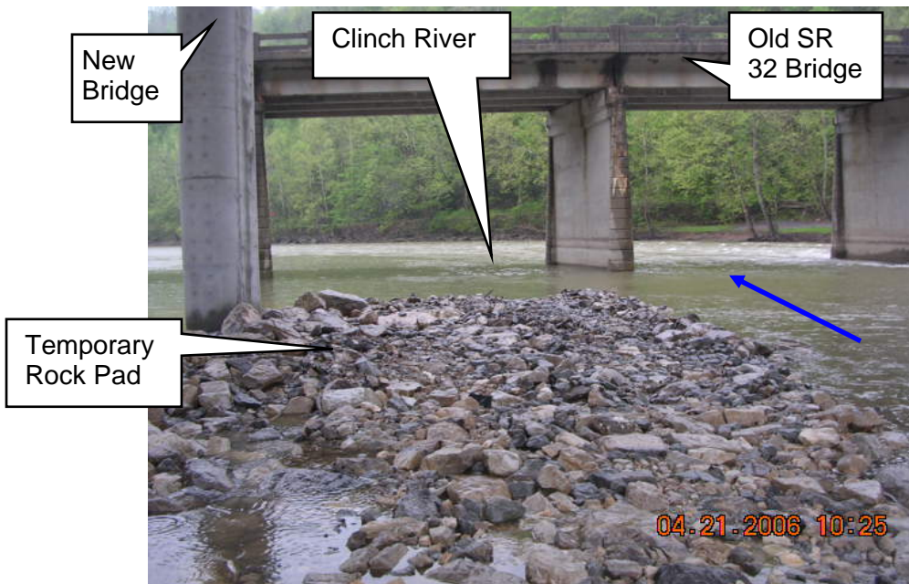
Photo 3. Temporary rock pad for bridge construction at Sta. 3+540 (both sides of centerline). View from south bank of the Clinch River looking southwest.
